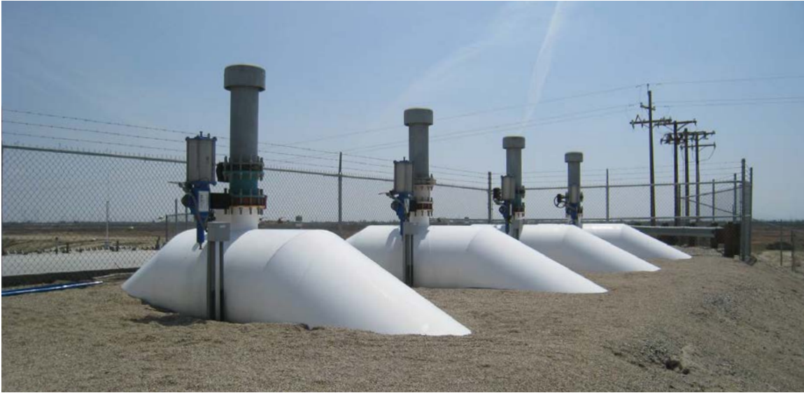
Pumps at the Kern Water Bank. (© Chris Austin)
