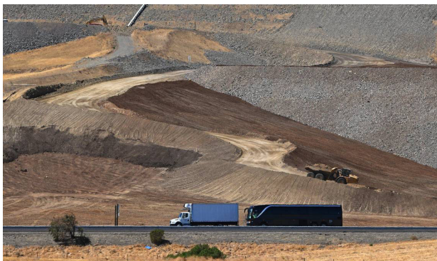
Traffic passes along Highway 152, bottom, as construction continues in the first phase of improvements at the B.F. Sisk Dam west of Los Banos Friday, Aug. 16, 2024. ERIC PAUL ZAMORA ezamora@fresnobee.com
