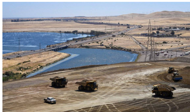
Looking down from the top of the B.F. Sisk dam, heavy machinery is seen preparing the ground with O'Neill Forebay and Highway 152 seen in the background Thursday, Aug. 8, 2024 near Los Banos. ERIC PAUL ZAMORA ezamora@fresnobee.com
