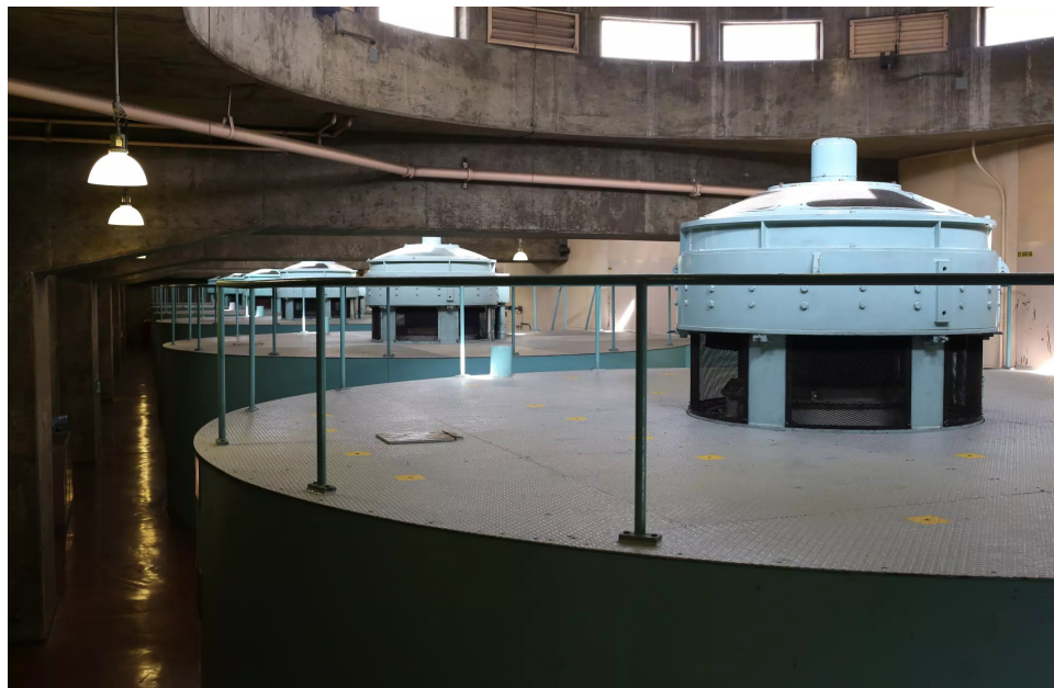
Motors at the C.W. “Bill” Jones Pumping Plant in Tracy, Calif. (Katie Falkenberg / Los Angeles Times)
